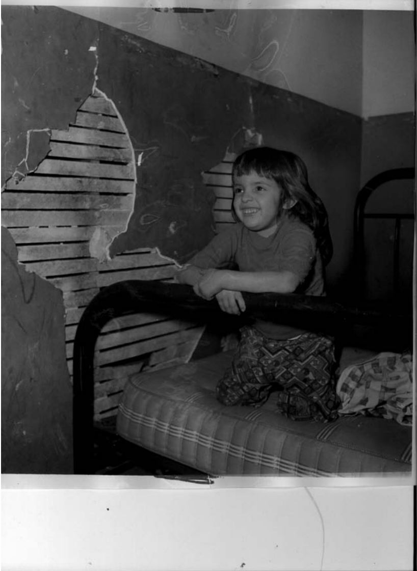
FIGURES 3A. Children at risk, 1960s. During the War on Poverty, peeling and chipping paint became a symbol of urban blight and social inequality. Community activists and housing reformers were critical in pressing for improved conditions. Source: (a) Chicago Tribune , February 3, 1966, reprinted with permission;
